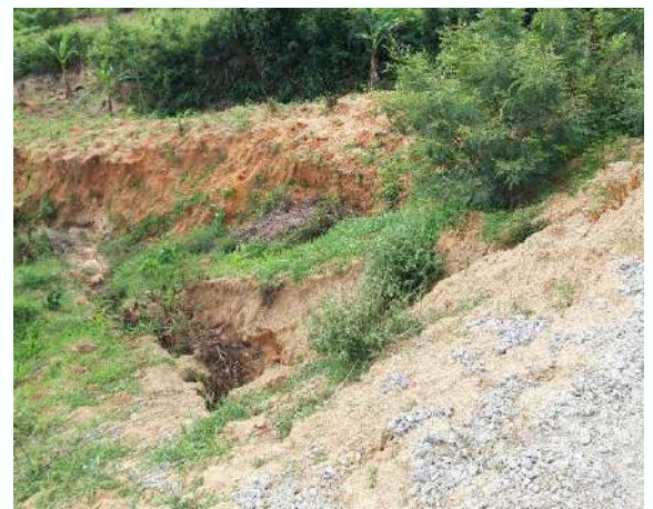
Collapse of slopes after a wet period
