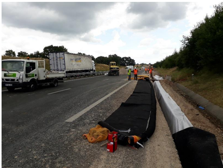
Installation of the collecting pipe inside the filter sleeve thanks to a pulling wire industrially incorporated inside the sleeve
