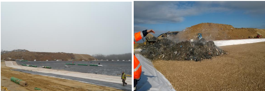
Figure 3. Installation of the geotextile reinforcement (Geoter® FPVA) and laying down of waste
