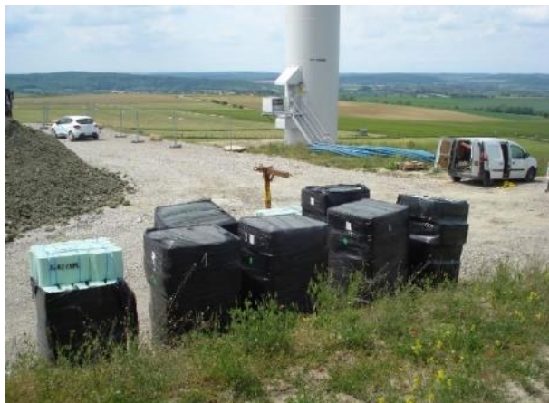
Figure 6. Storage for a 200 m (656 ft.) long and 4 m (13 ft.) high retaining structure
