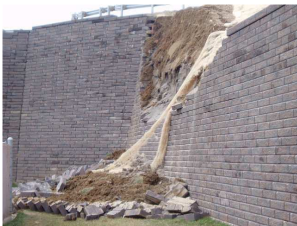
Figure 1. Example of a MSE wall failure
