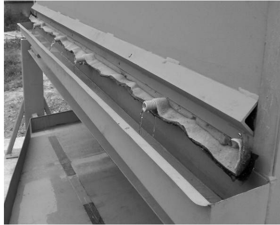
Picture 3: Drained water collector
