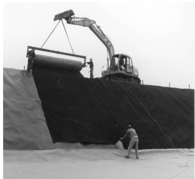
Figure 12. Geocomposite drainage layer with filter guaranteed anti-UV for two years
