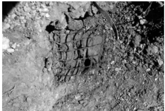
Figure 8. State of the top soil securing geogrid
