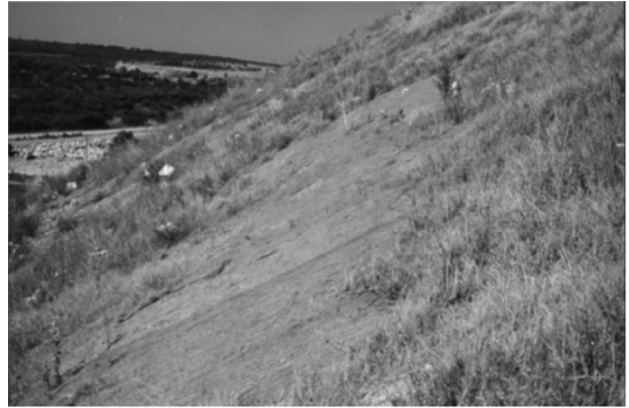
Figure 7. State of section n° 2 over a year later
